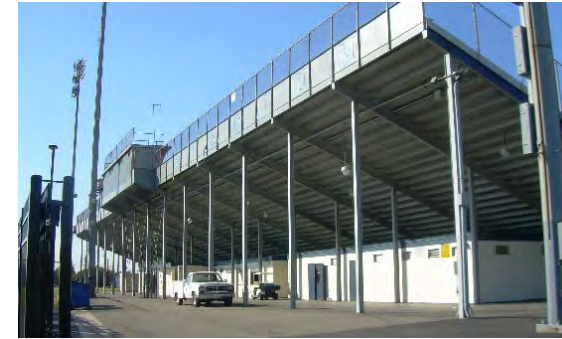
Stadium is in need of renovation
