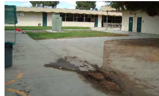
Poor concrete/asphalt conditions campus wide.
