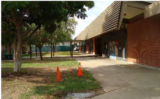
Major drainage/ponding issues in campus courtyards.
