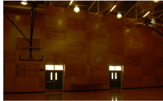
Gymnasium floor needs to be refinished.
