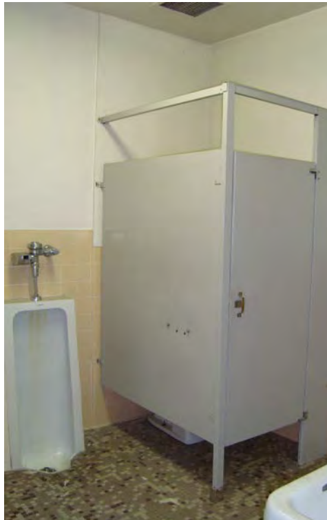
Provide ADA accessible restrooms.
