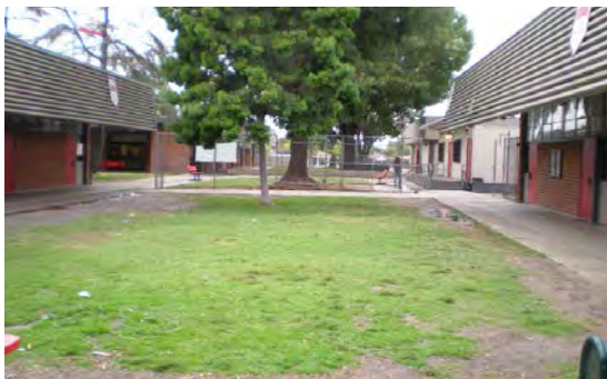
Courtyard landscaping and irrigation need to be replaced.
