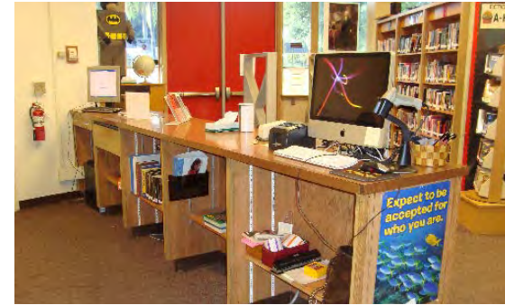
Library in need of renovation.
