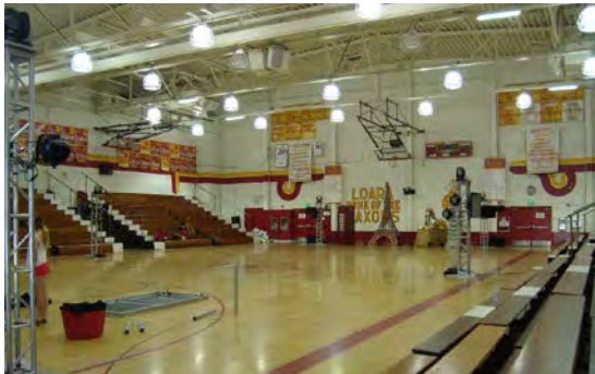
Poor ventilation in gym needs to be addressed.
