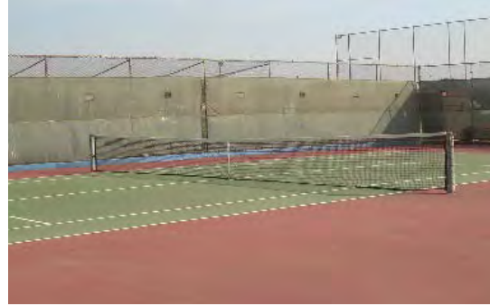
Tennis courts need resurfacing.
