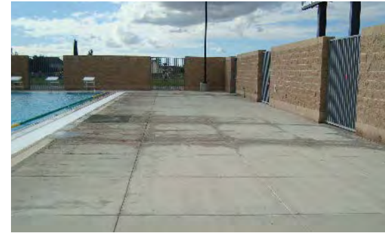
Pool in need of modernization; deck resurfacing.
