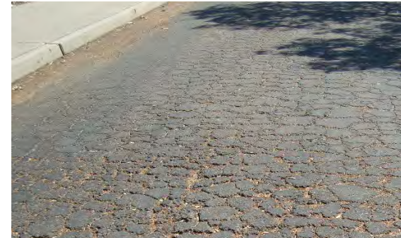
AC paving poor at parking lot.
