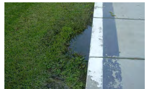
Address flooding/ponding issues between buildings.
