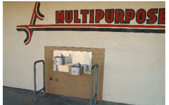
Interior/exterior of buildings need to be repainted.
