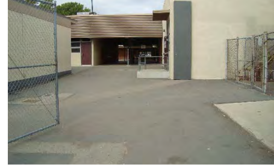
Poor asphalt conditions throughout campus.
