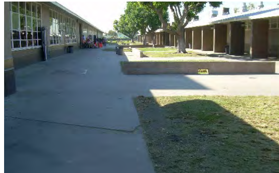
Overall paving in poor condition across campus.
