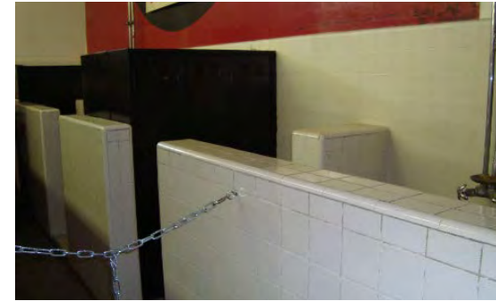
Locker rooms in need of expansion/consolidation.
