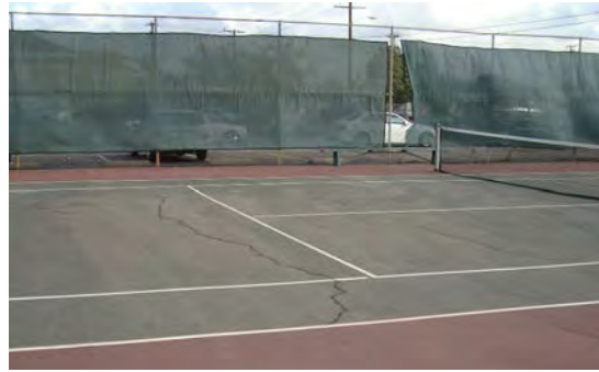
The tennis courts need to be replaced.
