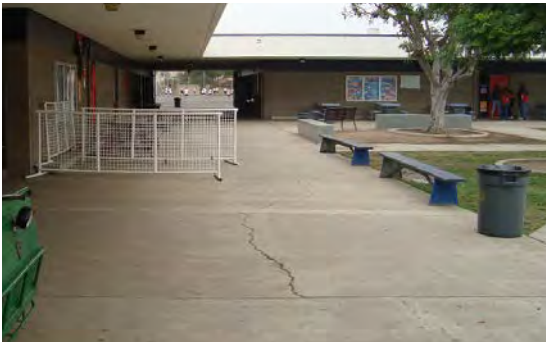
Campus concrete is in poor condition, especially at quad.
