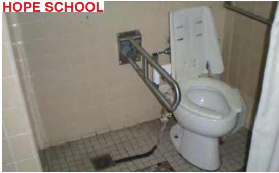
Additional specialized toilet facilities are needed.
