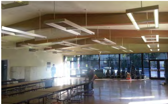
Cafeteria in need of upgrade and expansion.
