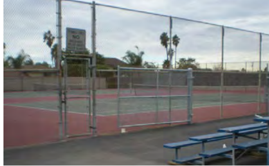
Need to refurbish tennis courts.
