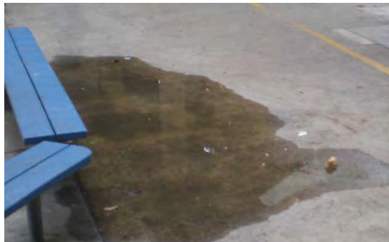
Ponding/drainage issues need to be addressed.
