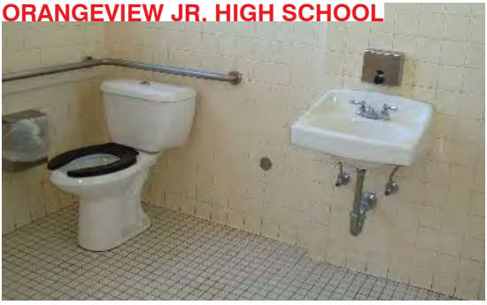
Campus restrooms are in need of an upgrade.
