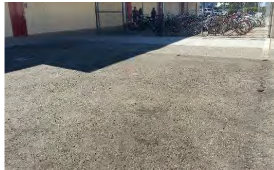
Campus-wide paving is in poor condition.
