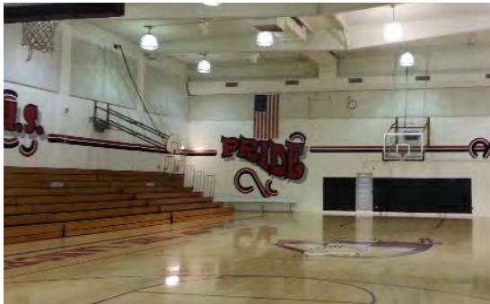
Gym floor and bleachers need to be replaced.
