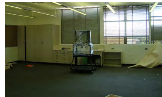
Standard modernization needed in classrooms.
