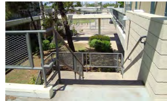
Accessible handrails needed at stairs and at upper level.
