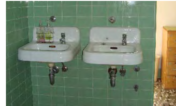
Restrooms are in need of upgrades.
