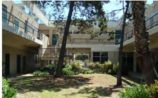
No ADA access to upper level. Provide elevator.
