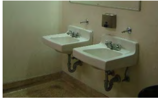
All restrooms need renovation.
