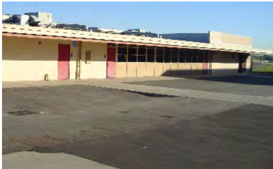
Existing paving in poor condition throughout campus.
