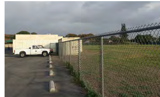
Need to replace fencing throughout.
