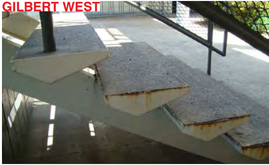
Stairs in poor condition.
