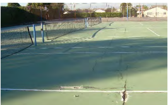
Tennis courts require resurfacing and/or replacing.
