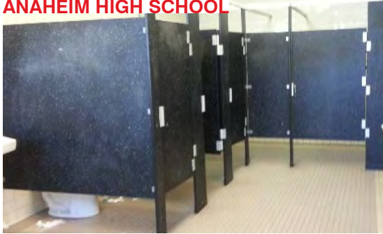
Restrooms need to be upgraded.
