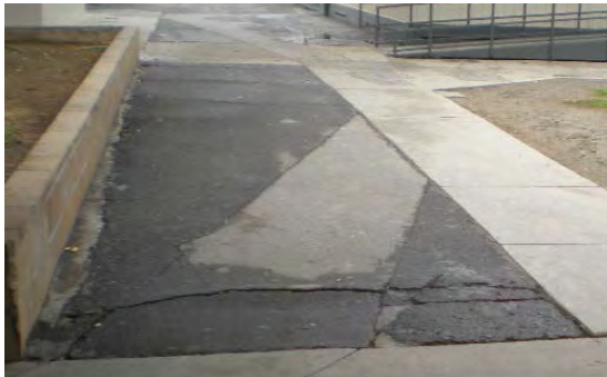
Campus wide asphalt paving in poor condition.
