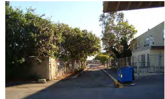
Drainage issues at the south of campus.
