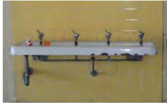
Accessible hi-lo drinking fountains are required.
