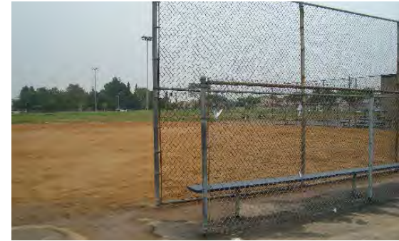
Softball infield and backstop are in poor condition.
