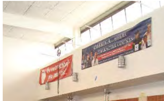
Replace leaking clerestory windows in locker rooms.
