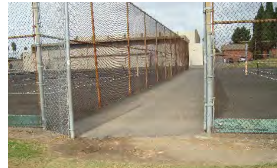
New fencing required in various areas.
