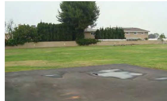
Minor ponding and flooding issues on campus.
